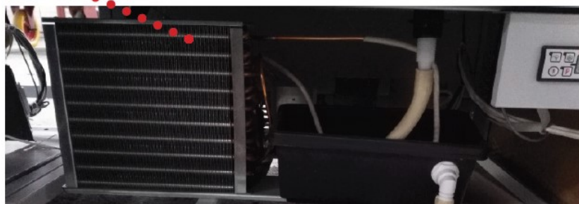
location of the condenser
