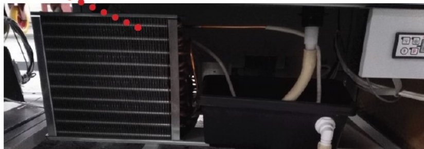
location of the condenser
